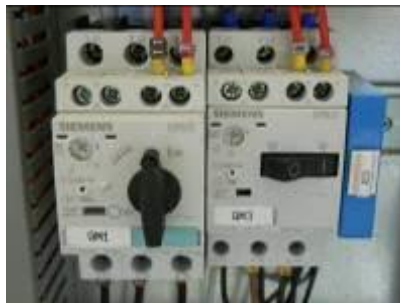
Picture 19 – All circuit brakers ON
