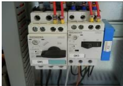
Picture 15 – pump breaker On
