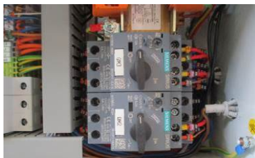
Picture 12– pump breaker On
