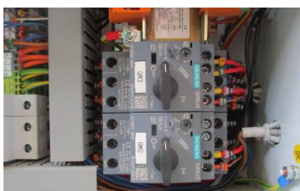
Picture 8 - Circuit Breakers
