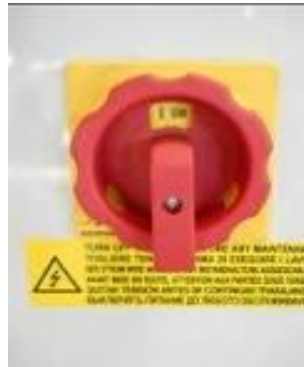
Figura 16 – Interruptor general en ON
