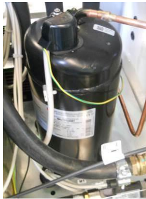
Picture 21 – Compressor placement
