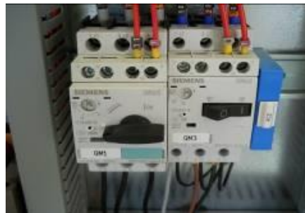
Picture 15 – pump breaker On
