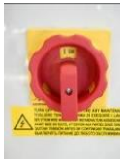
Picture 16 – Main switch ON
