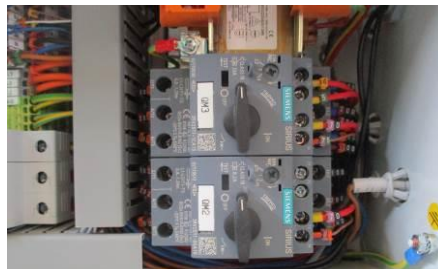
Picture 8 - Circuit Breakers
