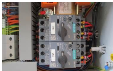
Picture 12– pump breaker On
